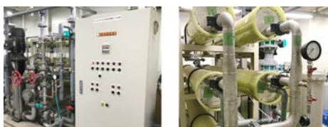
Reverse Osmosis (RO) Filtration Equipment
