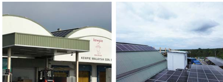
Photovoltaic panels installed at the Kewpie Malaysia Sdn. Bhd.
