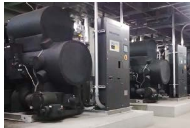
Ammonia freezer units
